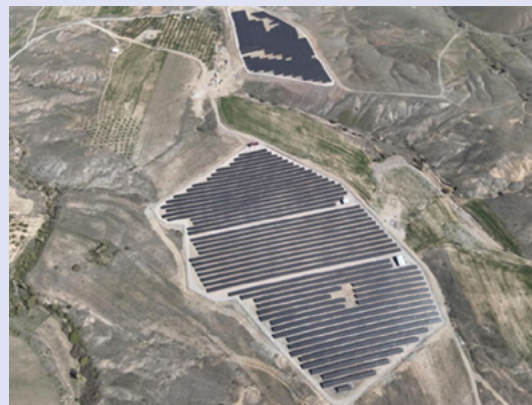
AISIN TURKIYE SOLAR POWER PLANT
